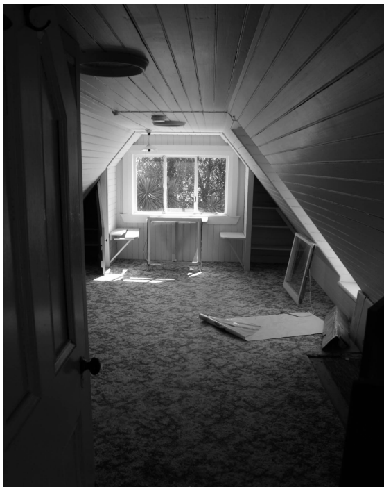
Figure 8 (left). Servants' bedroom, looking north-east. The window at the end is a 20 th century addition; the gable space formally held the chimney for the kitchen range below.
