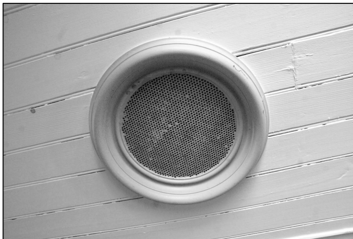
Figure 12. Plain ceiling ventilators in the attic Rooms I and H.
