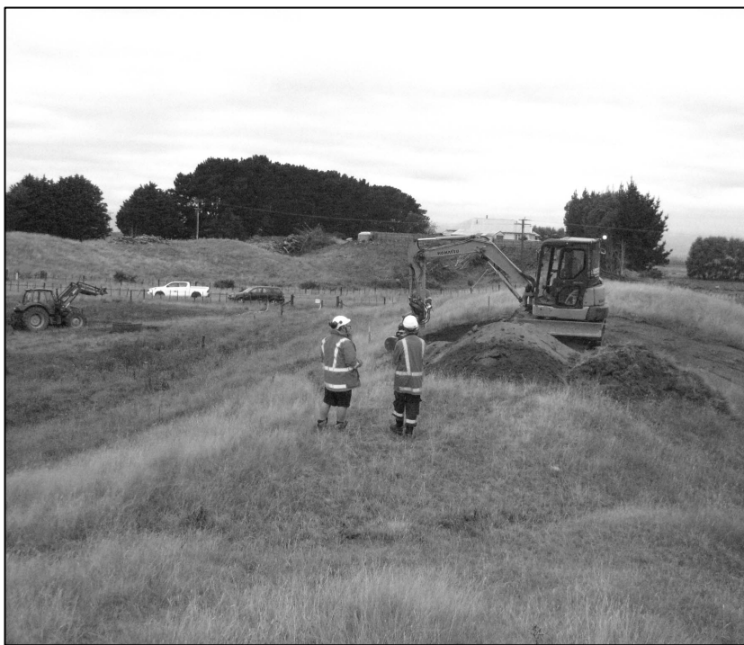
Eel channel S24/90 in the foreground, near Whirokino south of the Manawatu Bridge on SH 1.
