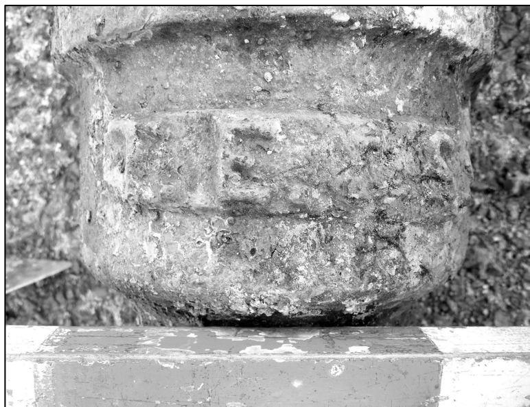
Embossed collar of cast iron 'T.E. & S.' pipe from Oamaru (Peter Mitchell).
