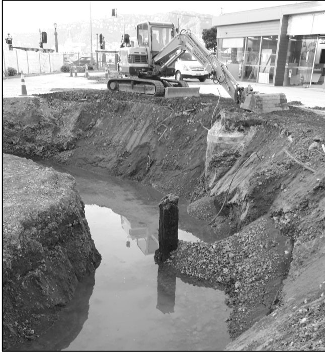
A pile of the 1890s Loan and Mercantile building in Wellington (Mary O'Keeffe).
