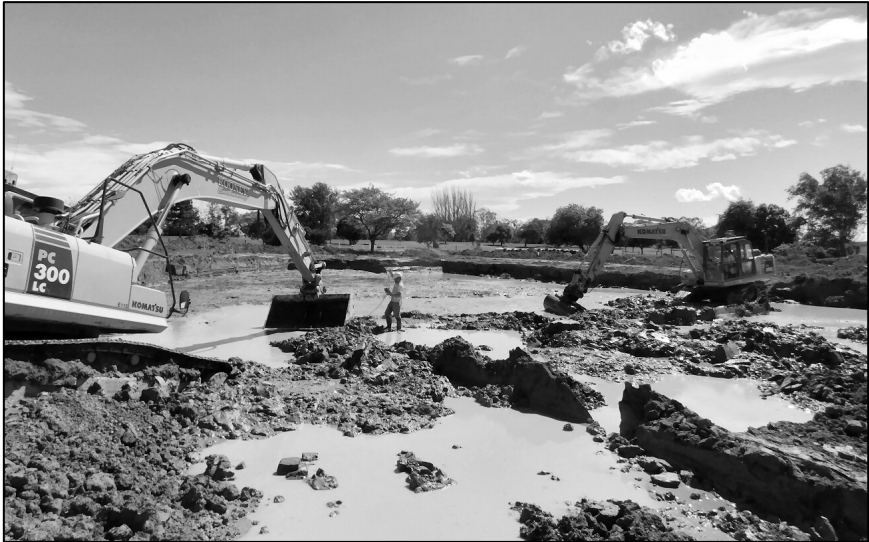
Ground conditions in Kaiapoi East sometimes make monitoring difficult (Jeanette McIsaac).
