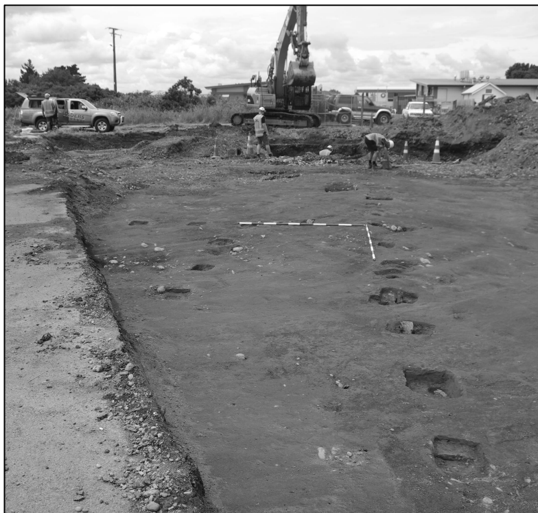
Post hole alignments delineating the southern corner of the Criterion stables, Bulls. Scales 2.0m (Subsurface Ltd, 2018)
