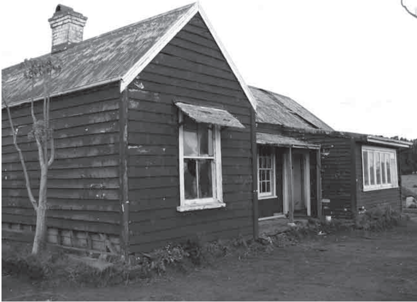
Figure 2. The front of the house from the southeast corner. The Phase III addition is in the foreground. The verandah may be a later addition to the original cottage.
