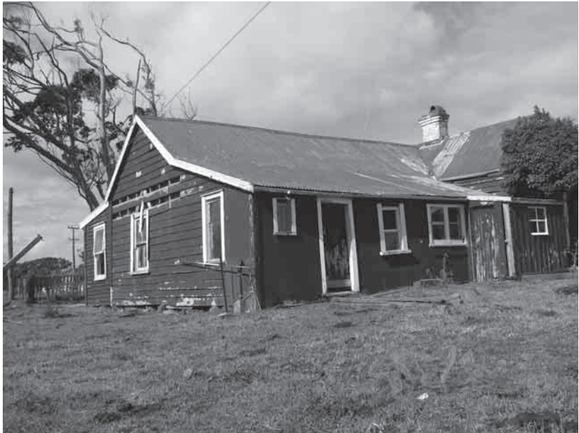
Figure 1. Scott House showing the north and west side prior to excavations starting. The main roofline in the centre is that of the original Phase I cottage and the room added on the north in Phase II. The lean-to is also Phase II. Wooden shingles were present under the roofing iron on these parts of the house. On the right, with the brick chimney, is the Phase III addition to the house.
