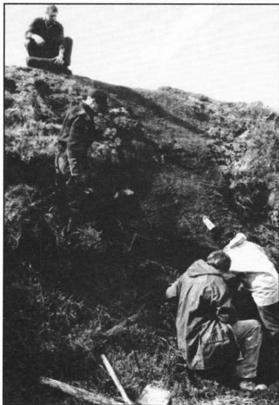
Figure 5. Rolls of instant turf being laid and cut to fit and secured in place using popsicle sticks (south side rut).
