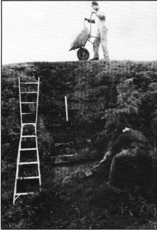
Figure 3. View showing the retaining boards in position and backfilling well underway using rotten turf (west side)
