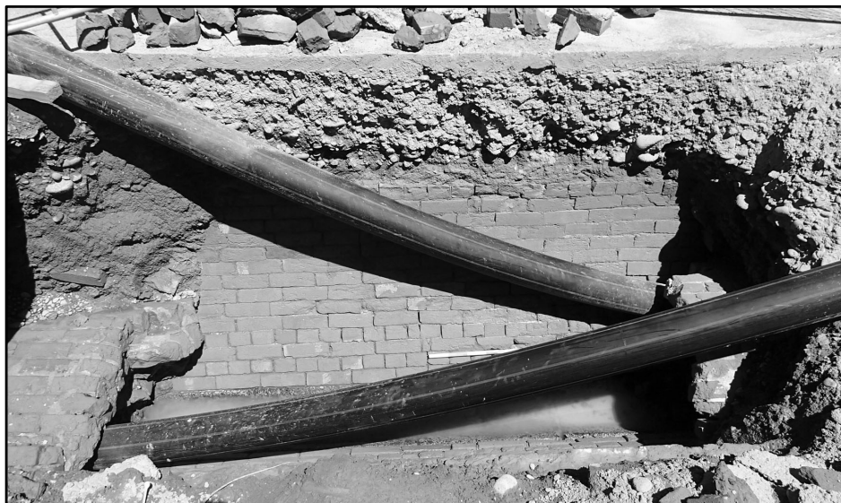
A 19 th century brick sewer containing 21 st century infrastructure in Tuam Street, Christchurch (Hamish Williams).
