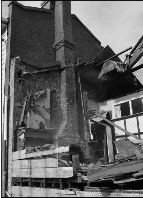
Demolition of the Arthur Street shop, showing the old chimney and fireplace (Andrea Farminer).
