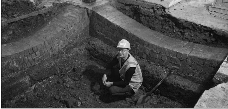
Matt Schmidt of HNZ and R.A. Lawson's inverted arch foundations under the John Colours building in Crawford Street, Dunedin (Otago Daily Times).
