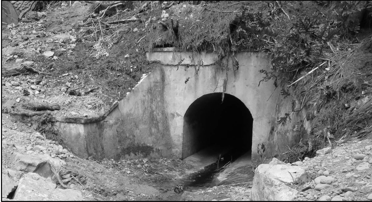
One of the restored culverts on the Rimutaka Rail Trail (Victoria Grouden).
