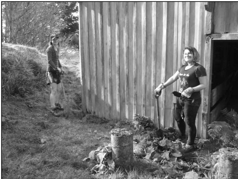
Figure 5. Clearing the drain around the west wall of the byre. This view also shows the original board and batten cladding.
