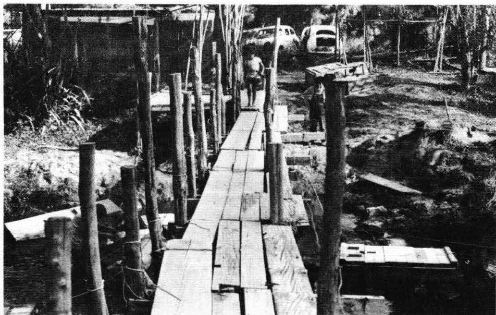
Figure 3: The awa looking along the walkway to the working platform and living shelter beyond.
